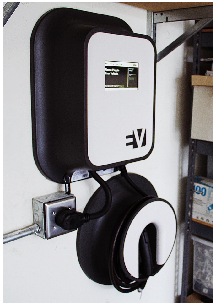
ECOtality's Blink Level 2 Home Charging Station (Plug-In Version) Installed in an EV Project Participant's Garage.
